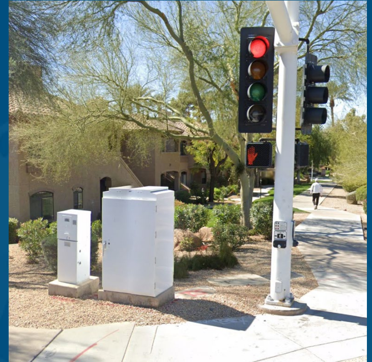
Existing Traffic Signal Equipment
