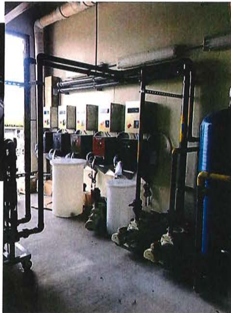
Right: New on-site generation system
