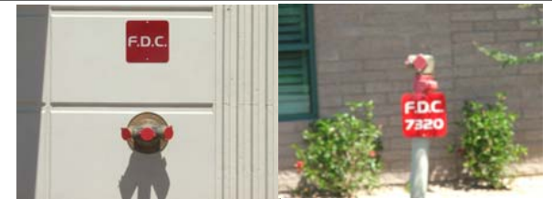
Fire Department Connections clearly marked
